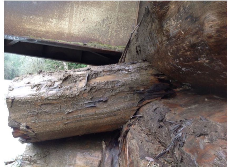
top tieback upstream right bank completely sheared off
