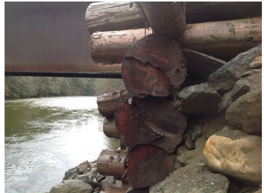
top crib log does not appear to have shifted - monitor
